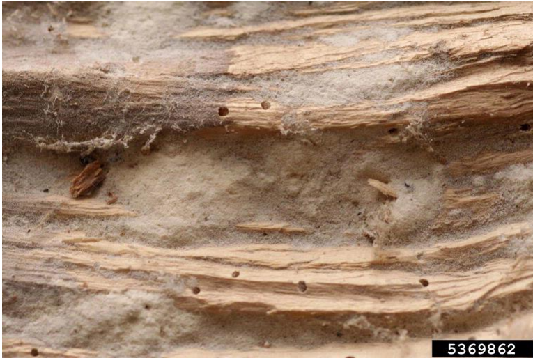
Wood damage from powder post beetles.
